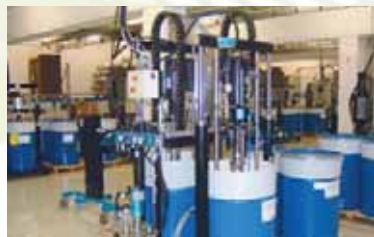
Extrusion pumps 23:1 ratio, used in multi component skids to transfer silicon
