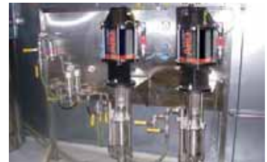
4-ball piston pumps 4:1 ratio, installed on a paint formulation process
