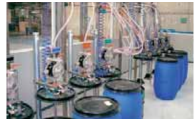
1/2" diaphragm pumps installed in a colouring process
