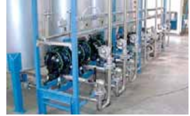
1 1/2" aluminium diaphragm pumps installed to feed a chemical reactor
