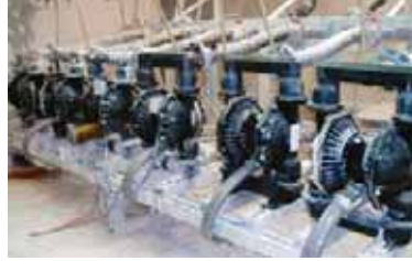
3" diaphragm pumps mounted on a skid to transfer clay in a ceramic manufacture
