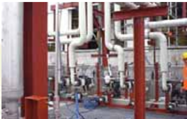
2" stainless steel diaphragm pumps assembled with PVDF pulsation dampeners used to download hydrofluoric acid
